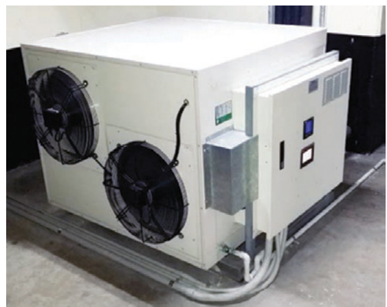
Air Change's PoolPac Plus installed in Avanti Apartments' plant room.
