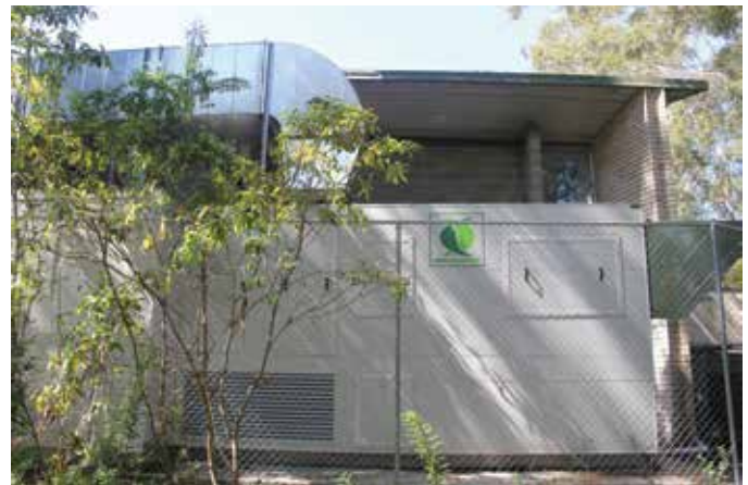
The PoolPac Plus Unit at Galston Aquatic and Leisure Centre in Sydney.
