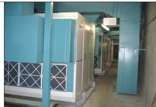
Four split construction, sandwich Air Change PoolPac units, with generous access doors on two sides, fit neatly into the existing plant room.
