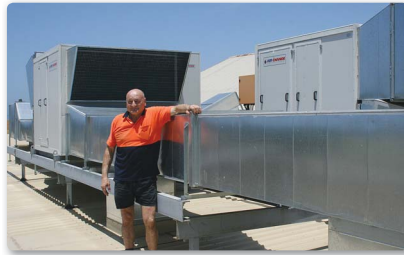
Insulated ducting takes 9,000 litres of 100% conditioned fresh air per second into the Anita Theatre during performances.
