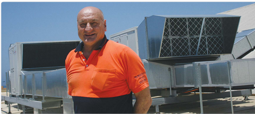
The proud owner of the beautiful Anita's Theatre at Thirroul, John Comelli, in front of the roof-mounted Air Change system.
